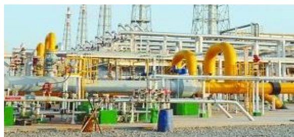
Figure 1. Pretreatment process of produced water in natural gas treatment plants.
